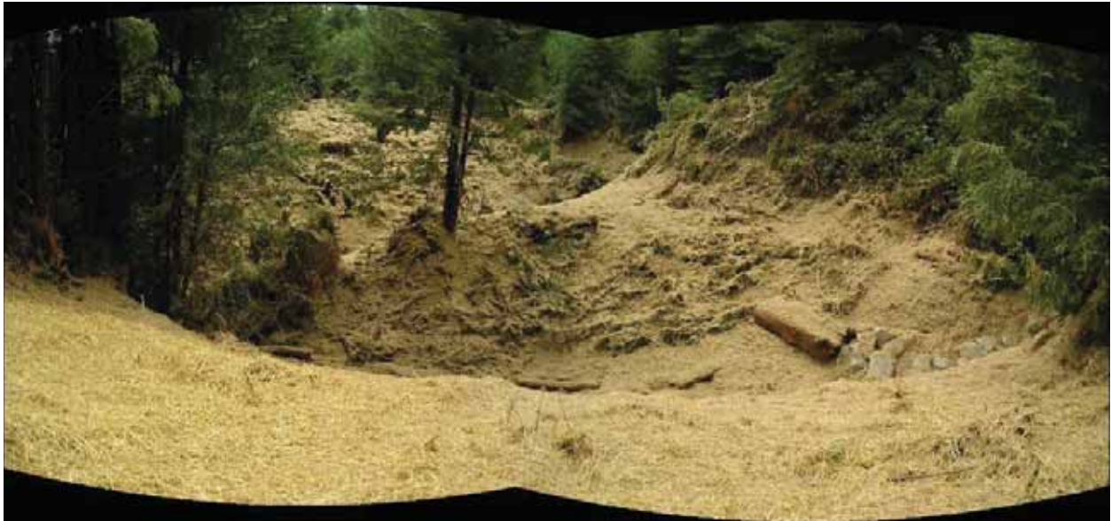
The same two crossings after the restoration work was completed. Note the rock protecting the upstream part of the channel and the slash (small trees and limbs) providing bank stabilization. The larger wood chunks were excavated from the crossing. Straw covers all bare soil for erosion control.
